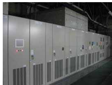
Electric double-layer capacitor equipment
