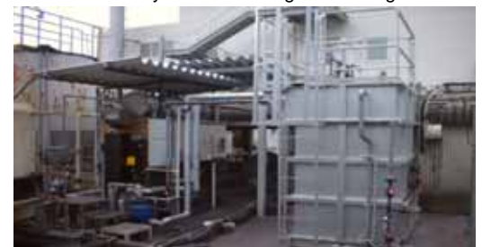
Low pressure dewatering drier
