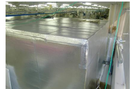
Insulation of burn-in facilities
