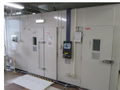
Highly efficient chamber (HQs / Tokyo Plant)
