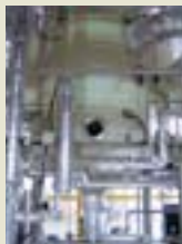
Alkali compaction equipment
