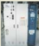
PFC removal equipment
