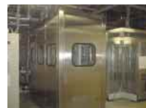
A sulfuric acid recycling facility (Fujitsu Iwate Plant)
