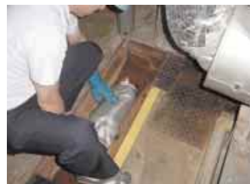
Placement of sandbags along the upper part of a wastewater ditch to prevent drainage into sewers
