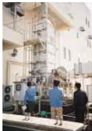
A facility management survey of Kyushu Fujitsu Electronics' waste gas cleaning facility
