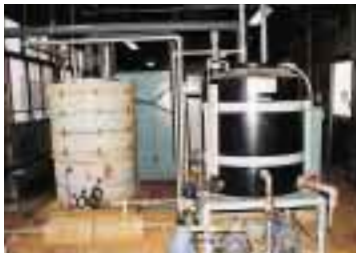
Purification equipment (Kawasaki Plant)
