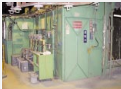
Solvent recovery equipment (Akashi Plant)
