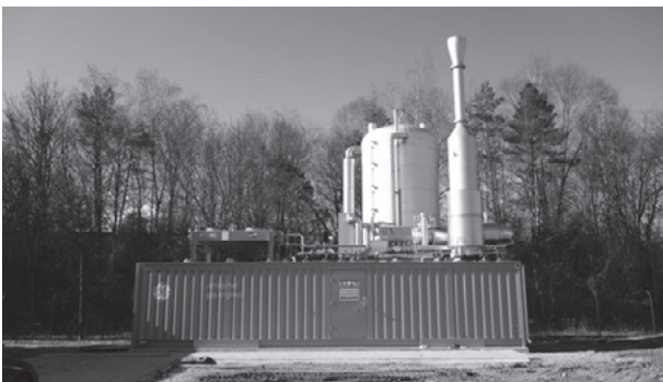
Figure 7 CHP in Augsburg.
