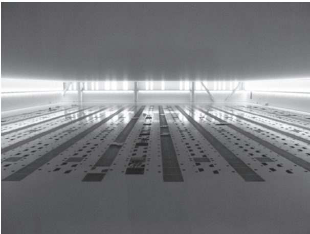
Figure 1 Third-floor computer room (before computer installation).
