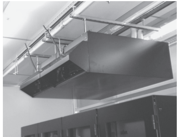
Figure 4 Local air-conditioning unit.
