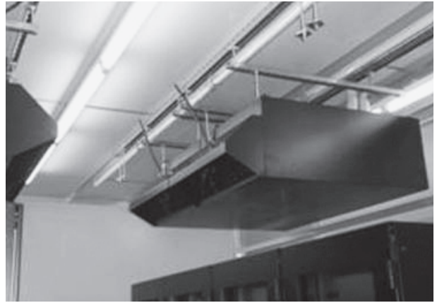
Figure 5 Local air-conditioning system.
