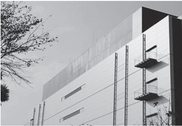
Figure 6 Photovoltaic power generation panel (vertically installed portion).
