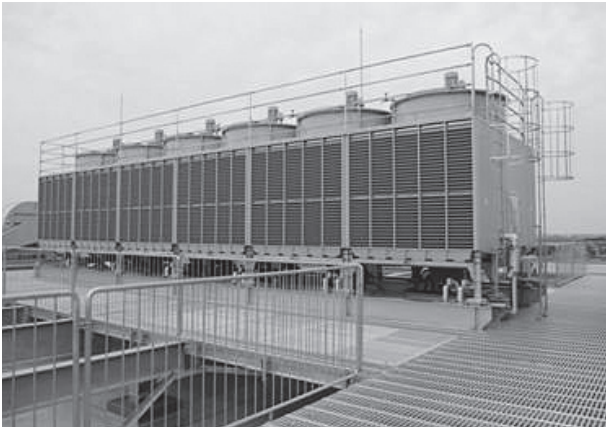
Figure 4 Cooling tower for free cooling.
