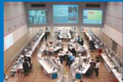
Integrated Control Room of Tatebayashi System Center
