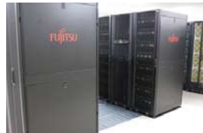
New supercomputer system
