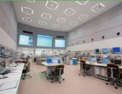
Control room of the Fujitsu Tatebayashi System Center, Japan's largest outsourcing center
