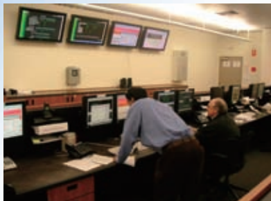
Control room of data center operated by Fujitsu Australia
