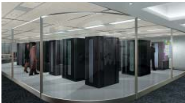
The server room at our Platform Solution Center in Tokyo
