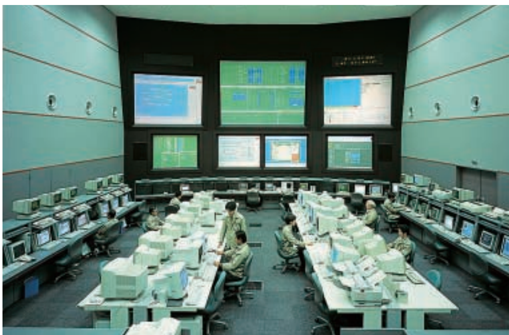
Tatebayashi System Center's integrated control room
