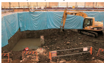
Contaminated soil removal from an underground storage tank at the Suzaka plant
