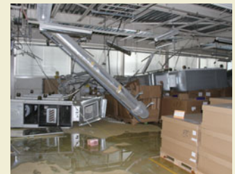
The damaged Fujitsu Isotec Plant
