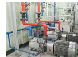
Pipe to return water to the chiller (blue pipes)
