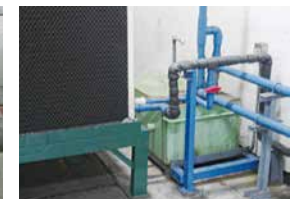
Close Loop Circulation (blue pipes)
