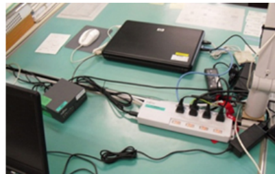
Connecting a gateway, a smart power socket and a notebook PC
