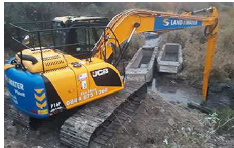
Dredging of a lagoon to act as a water basin (United Kingdom)
