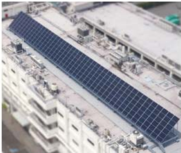
Photovoltaic Power Generating System
