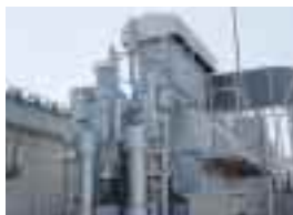
Improved organic chemical waste processing equipment (Aizuwakamatsu Plant)
