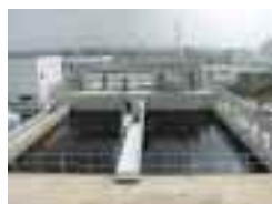
Copper-plating waste liquid-processing equipment
