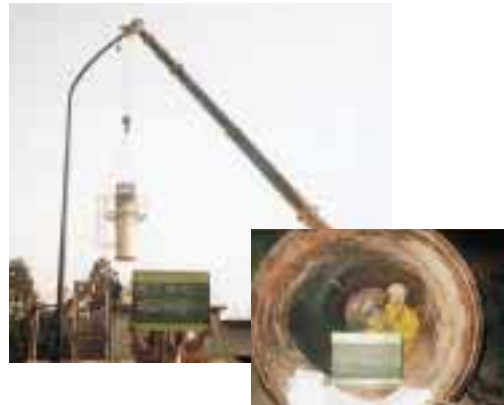
A decommissioned waste incinerator
