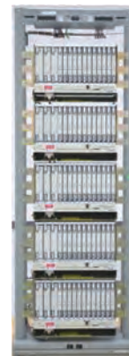
Preconfigured Rack Solution
