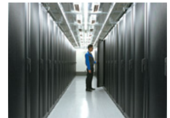
Pic.2 : One of the largest data centers in Japan, TISC's server room covers more than 3,300 m 2 .
