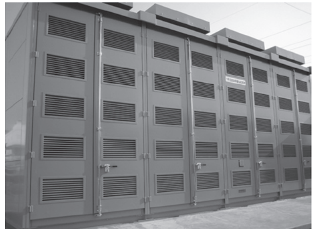
Figure 6 Introduction of NAS cell (Mie Plant).
