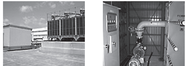
Figure 7 Introduction of free cooling system (Yamagata Fujitsu Ltd.).
