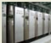
Small boilers burning natural gas
