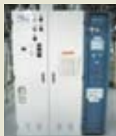
PFC removal equipment
