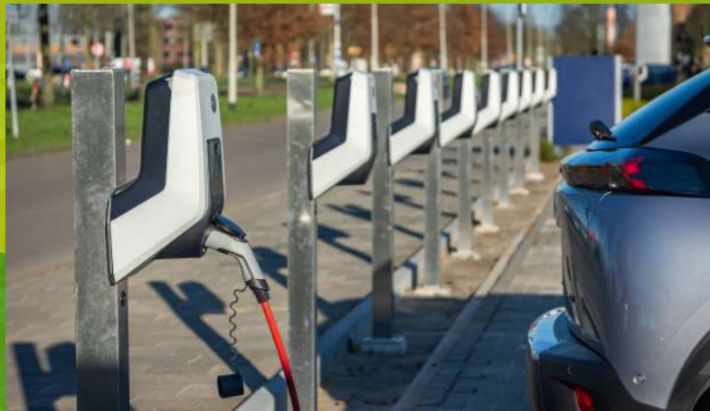
An electric car charging station in The Netherlands
