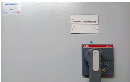
Switching Mechanism to enable Fujitsu Datacenter UPS to power local water pumps in the event of a flood (United Kingdom)
